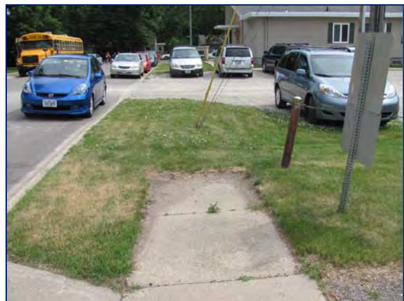
Sidewalk gap along the west side of Fern Avenue. Parents park on the west side and buses park on the east side. Parents cross the street with students.
