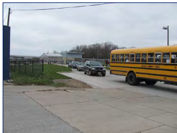
Vehicles waiting to exit onto U.S. Highway 63. Right-turn lane is not designed properly to provide adequate room for two exit lanes.
