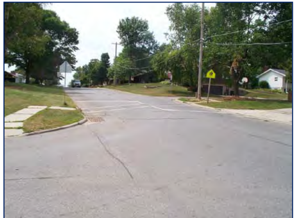
School crosswalk at 18th Street and Summit Drive. This crosswalk assembly is not the latest version of the school crosswalk assembly as shown in the MUTCD.
